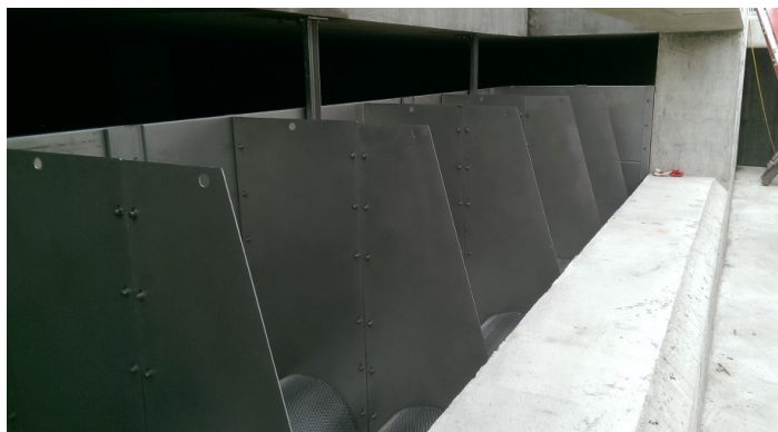
▲ Overflow weir—screen is positioned just below the weir on the inlet side.
