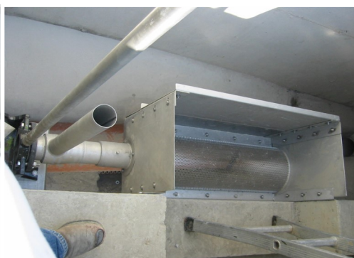
▲ Single screen arrangement, venturi and guide rail.
