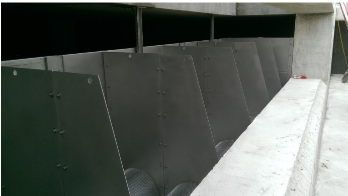
▲ Overflow weir—screen is positioned just below the weir on the inlet side.
