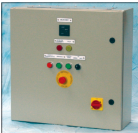
Typical Control Panel
